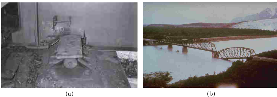
Figure 2.2: Unseating failures (a) of Pier 42 of Route 3 from the 1995 Kobe earthquake [19], and (b) of the "Million Dollar Bridge" over the Copper River outside of Cordova, Alaska was unseated during the 1964 Alaskan Earthquake [54]
