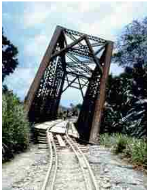
Figure 2.8: Lateral spreading around the foundations of a railroad bridge in Costa Rica during the 1991 Limon earthquake caused significant displacement of the structure [64].
