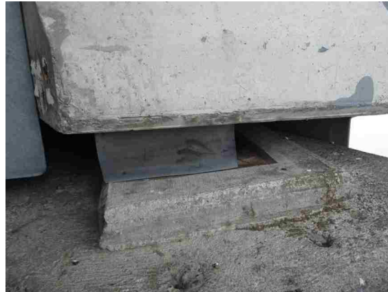
Figure 2.7: An unbolted elastomeric bearing supporting the Bridge Street bridge outside Christchurch experienced a sliding failure during the 2010 New Zealand earthquake [11].
