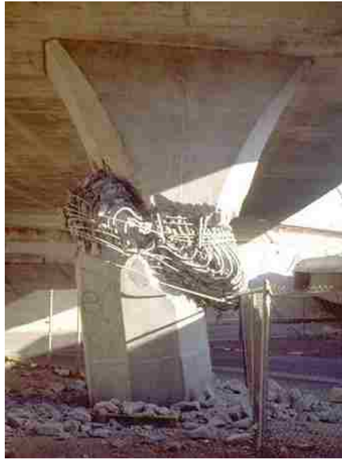
Figure 2.4: The flared piers of the Mission-Gothic underpass experienced shear failure during the 1994 Northridge Earthquake, likely after yielding of the longitudinal reinforcement reduced the pier's shear capacity [5].
